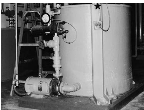
Reverse osmosis, Ósmosis invertida
